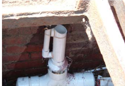
Figure 6. Example of inlet sampler to collect first flush samples (courtesy City of Baltimore)
