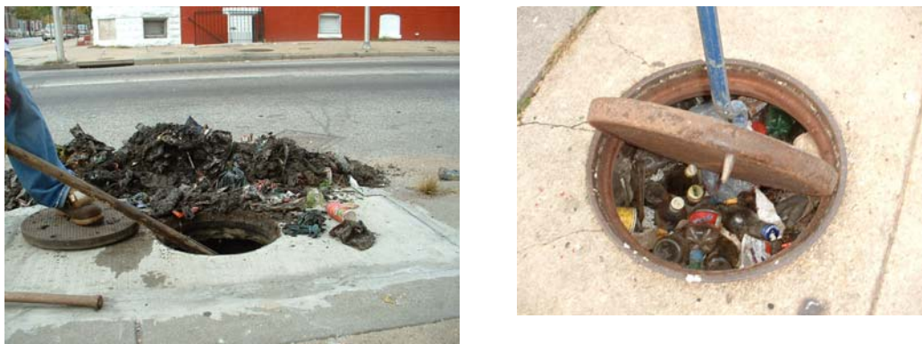
Figure 10. Example of material blocking storm drain inlet in catchment O.
